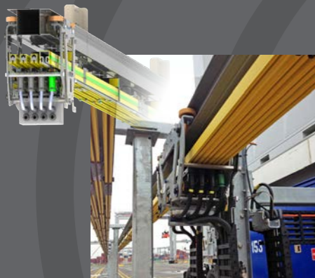
E-RTG with Drive-In L Solution and ProfiDAT®
